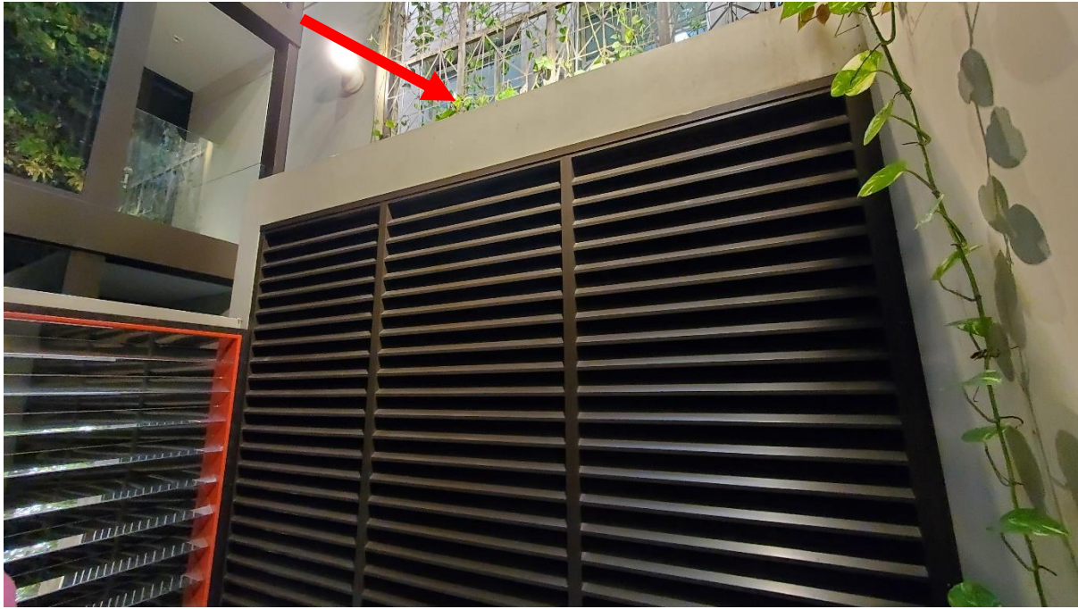
Figure 22: Internal view of level one resident balcony with the subject site terrace directly behind wall
